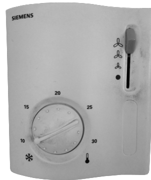
Figure 5.1: HVAC thermostat for controlling temperature setpoint.
