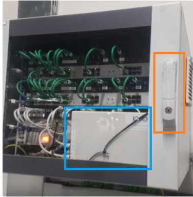
Fig. 6: COMSEC (in blue) on the locked airport switch cabinet (orange).
